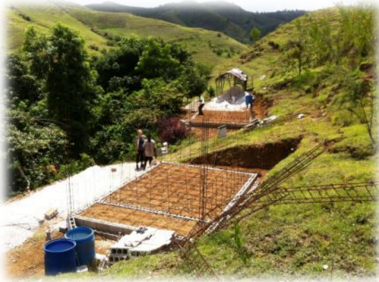
The contractor's crew works on the foundation, with vistas on Baby hill country in the background.
