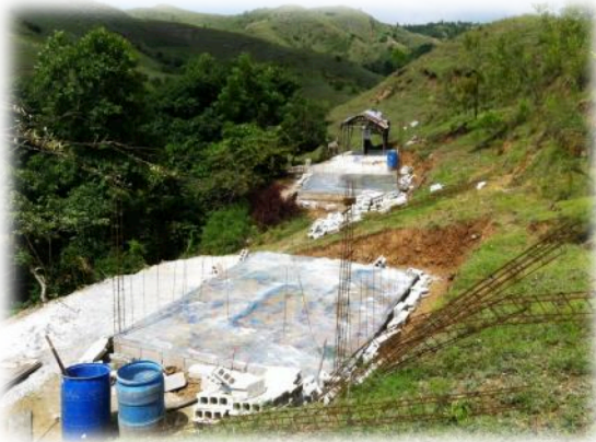
The families continue to stay involved by providing water to mix the concrete. This requires a good downhill walk to the river and back.
