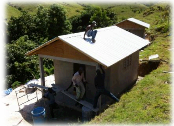
The contractor's crews are often assisted by visiting teams to install roofs.
